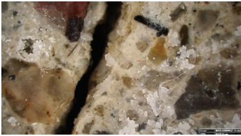
Magnified hairline crack in concrete
